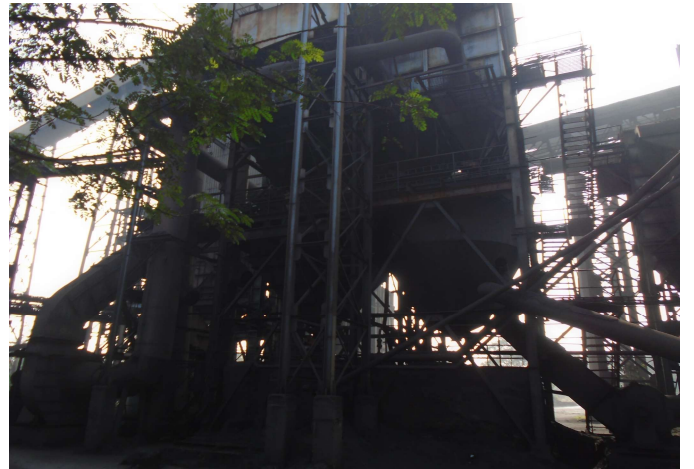
(figure 8: DRI New Bagfilters - Cap:33,200 m3/hr)
